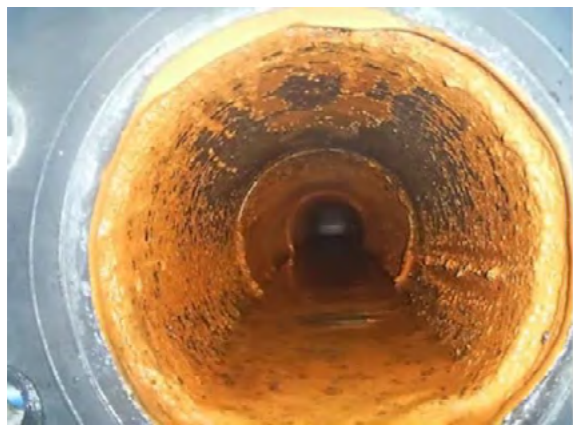
Figure 1 Pipes with severe corrosion
